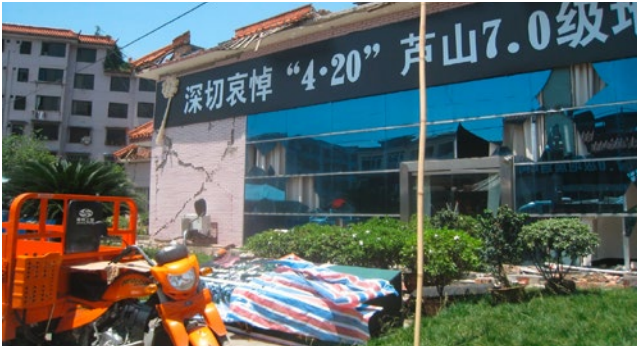
FIGURE 7 Damage of an office building during the Lu Shan earthquake
