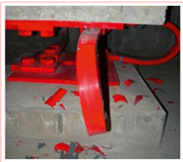
PHOTO 2 Deformation of U-shaped steel damper
