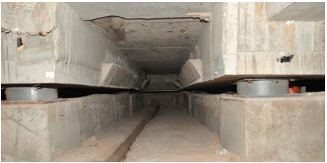
FIGURE 19 Base isolation system in a retrofitted school
